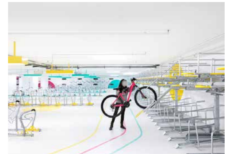
Figure 5.177 Bicycle storage system
