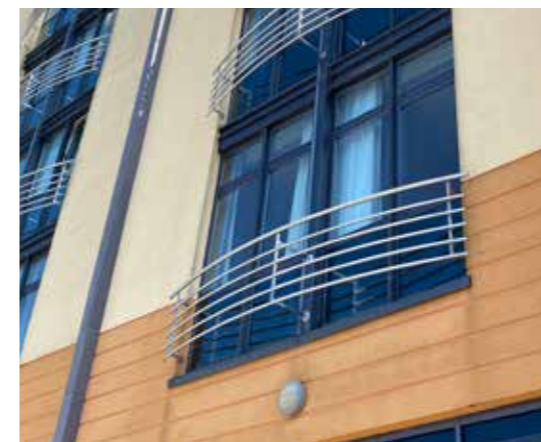
Figure 5.164 Example of not acceptable low quality 'stick on' detailing with a flat façade with no perceived depth
