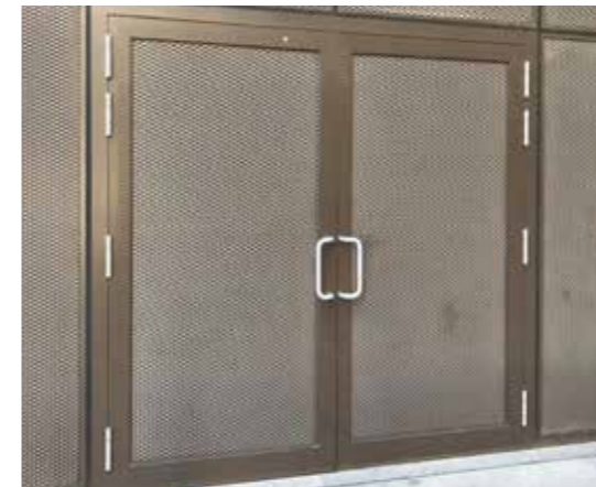
Figure 5.162 Example of detailing where ironmongery does not match overall material and tone compositions
