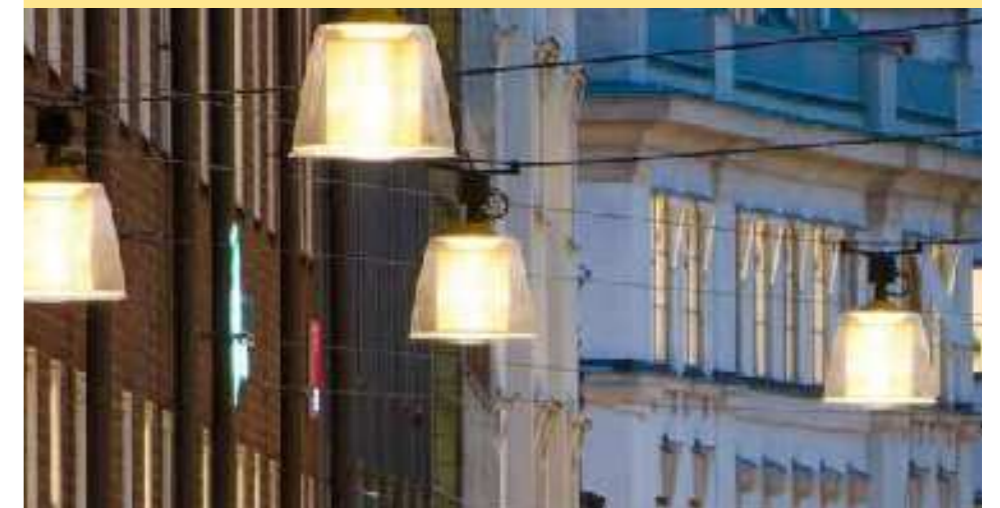
Figure 5.898 Catenary lighting to lanes
