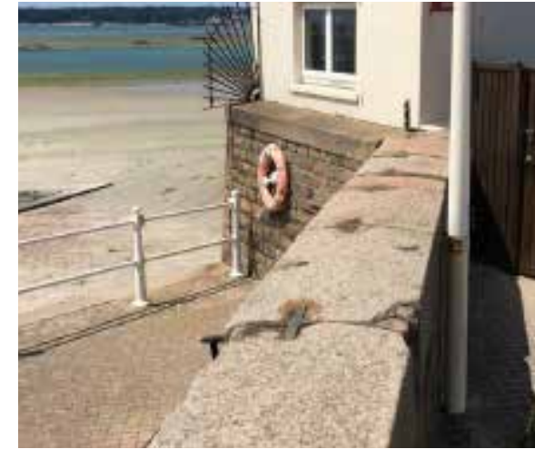
Figure 6.12 Site photo of barbed wire mounting points
