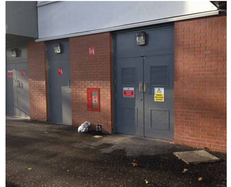
Figure 2.165 Plant rooms at ground floor creating unattractive facades. Servicing access requirements will greatly reduce capacity for street greening
