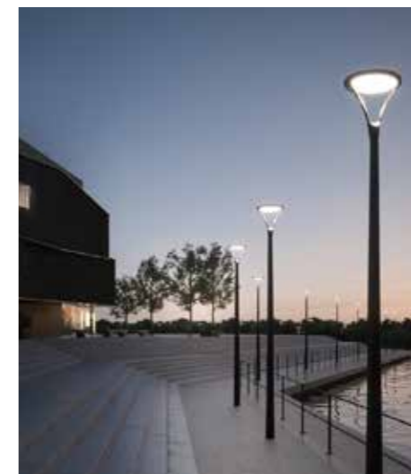
Figure 4.131 Pole mounted lighting to park
