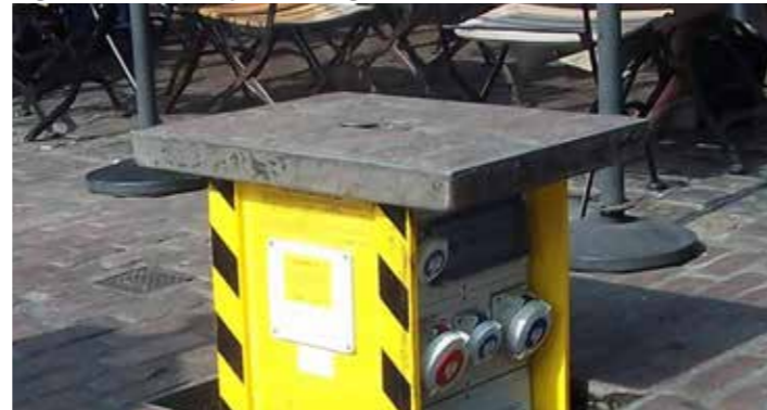
Figure 4.145 Pop-up power units for events
