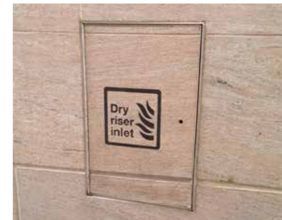
Figure 5.163 Example of a high quality coordination of façade with dry riser inlet
